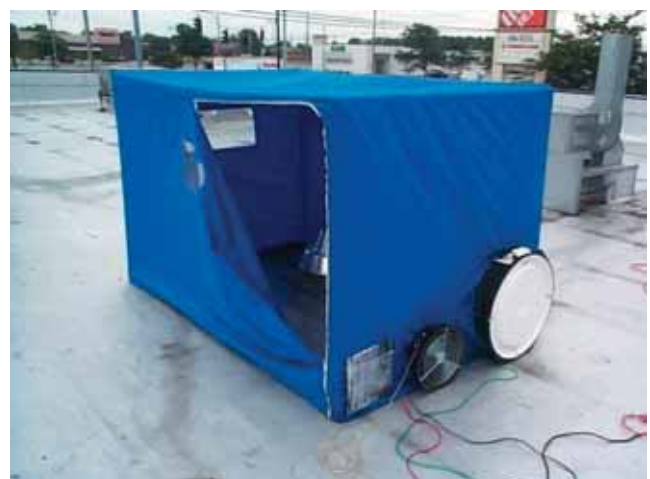
Figure 7 - Fan powered capture hood measuring flow from a rooftop exhaust fan. This method provides good accuracy but is limited to flows equal to or less than the flow of the calibrated fan. Photo courtesy of CDH Energy Corporation and New York State Energy Research and Development Authority.
