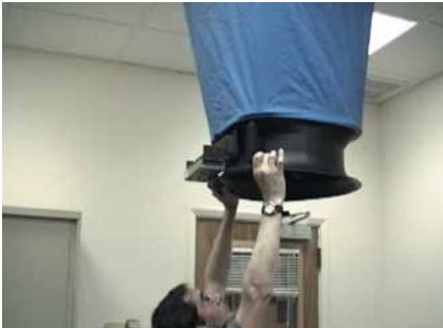
Figure 4 - Measuring total exhaust flows by summing flow through exhaust grilles (NOTE: This misses air leaks in the ductwork).
